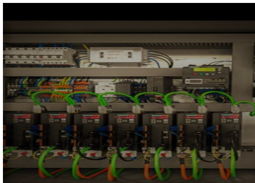
Fig 2: PLC control panel
